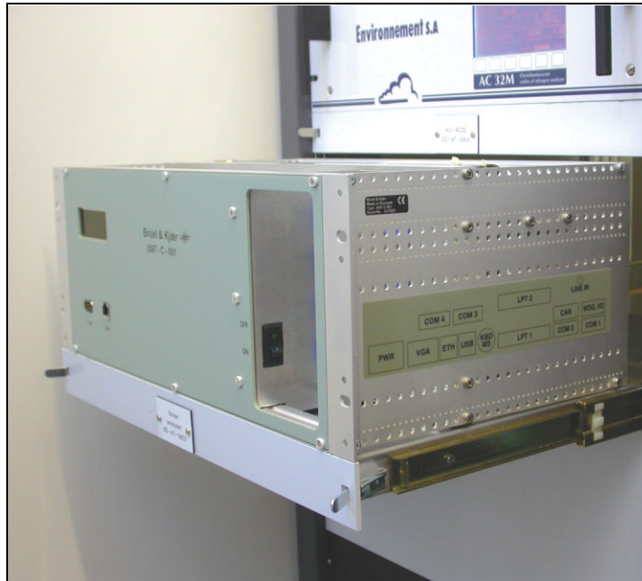
Fig. 4 Installation of Brüel & Kjær NMT at OMIFCO industrial site
