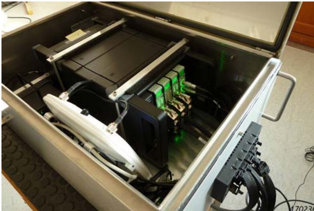
Fig. 7. LAN-XI modules installed in waterproof box
