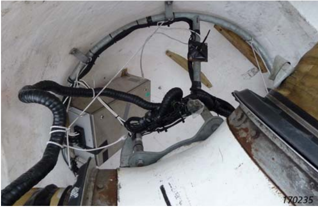
Fig. 8. Waterproof box mounted inside the spinner – cables not connected
